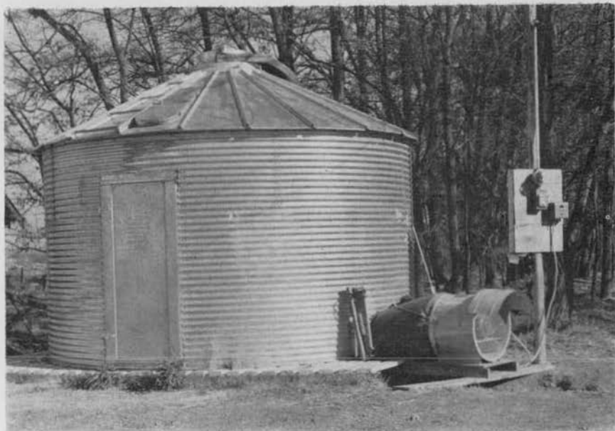
FIGURE 5. A 3-hp. axial-flow fan used for drying with unheated air.
