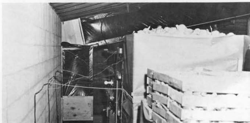
Figure 5. A rear-view of the same bins shown in Figure 4, showing the air duct and fan arrangement.
