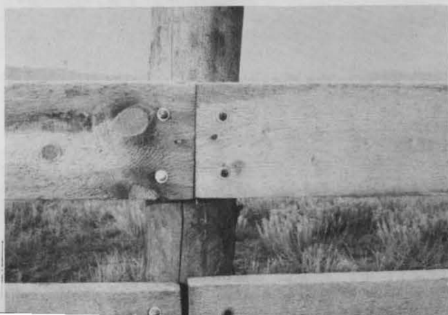
Figure 7 : A critical point in the construction of fences is the butting together of rails.
