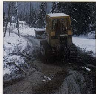
Winter thaws can happen. Don't take chances with soil disturbance and possible erosion. Expect to shut-down temporarily.
