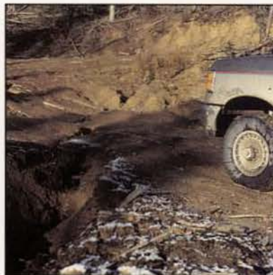
Before grading, it may be necessary to loosen hardened or deep rutted road surfaces. Ripper shanks on the grader are effective. Road repairs should occur before the wet season. Special attention is needed on steep slopes or curves where greater road surface wear occurs.
