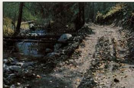
⊘ If grading produces excess material, feather it out or haul it away. Never side-cast material into streams. Avoid leaving a berm that channels water down the road unless it is routed into an effective vegetation filter that spreads it out and removes sediment.
