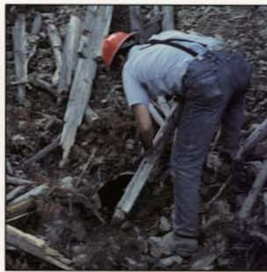
Hand, shovel, and chainsaw work are usually all that culvert maintenance requires. But don't delay! Delay in cleaning a blocked culvert or ditch can result in a damaged road that requires costly reconstruction.
