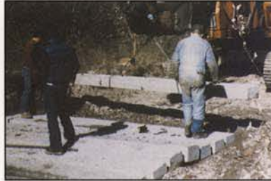
Concrete planks, fastened together and stretched across the stream bed, provide an improved ford crossing. Approximate cost: $100 per running foot, installed.
