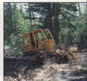
Road restoration includes pulling up roadside berms, ripping compacted areas, restoring natural drainage, and reseeding with appropriate grasses.
