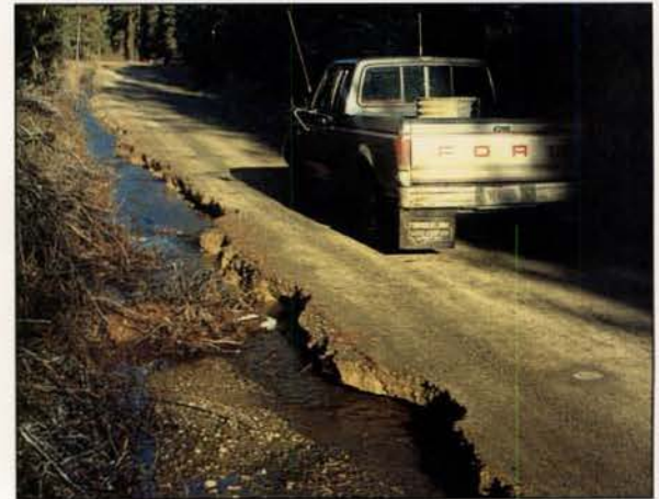
In contrast, the road drainage problem is the result of a plugged crossdrain culvert and washed-out catch basin.
