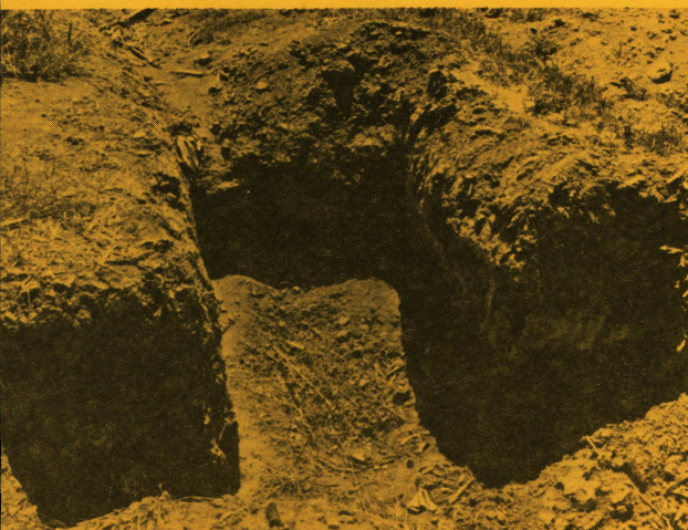
Fig. 5. A T-slot, dug in the tailditch with a backhoe, operates as a small settling pond to trap sediment washed off a field. T-slots will remove 50 percent of sediment that passes through but become ineffective when filled up.
