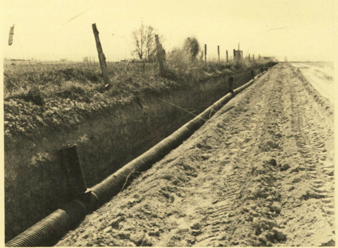
Fig. 6. A buried drain system assembled in a ditch made with a blade and ready to be covered.
