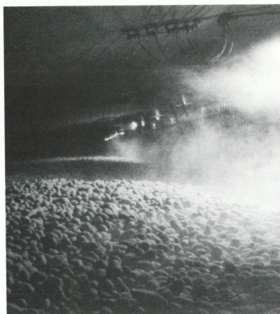
Figure 2. During treatment the CIPC aerosol is circulated throughout the potato pile by the circulation fans. The aerosol quickly fills the air spaces around the potatoes and inside the building as it is being deposited on the potato surfaces.
