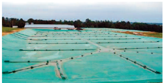
Figure 4. Covered-lagoon digester. (Source: http://www.epa.gov/agstar/anaerobic/ad101/anaerobic-digesters.html )
