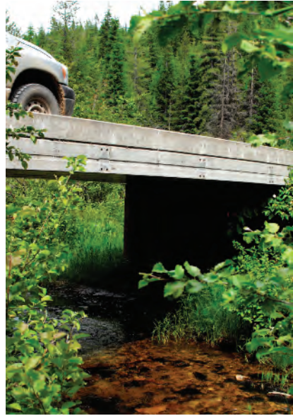
Bridges provide the best fish passage, have longevity, and require minimal maintenance.
