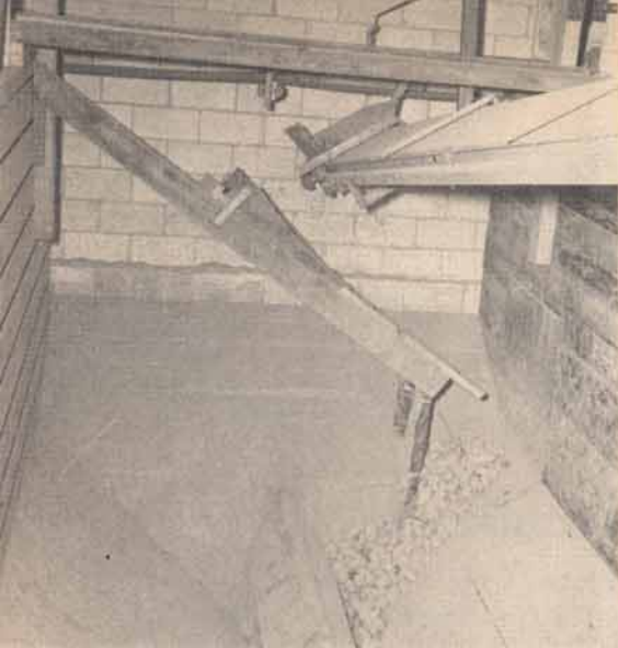
Figure 10.—An automatic-fill bulk storage bin. The inclined shelf at the back of the bin allows potatoes entering first to roll gently to the bottom. Potatoes are distributed in the bin by the tilted belt conveyor. All points of potato fall are rubber-padded to lessen injury.
