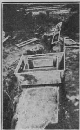
Figure VIII. —This picture was taken when the side walls had been placed and the forms for the top and man hole had been completed. This is the large size tank and the man hole was placed near one end.
