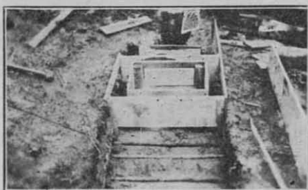
Figure X. —One inch of concrete was poured and then the reinforcement bars were laid across, about one foot apart.
