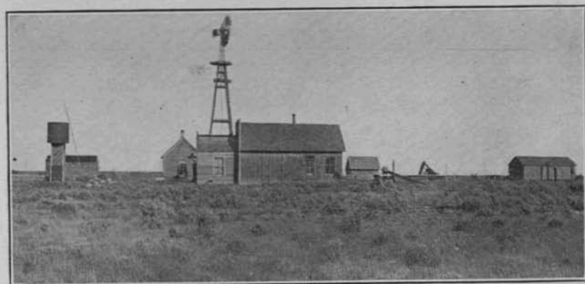
FIG. 25. This ranch has been occupied for fully ten years. The soil is excellent and supplied with abundant water for tree growing. A few cuttings from a neighbor's cottonwood trees could have been so placed years ago as now to furnish abundant shade, shelter and fuel, at the same time enhancing the value and attractiveness of the place and contributing immensely to the comfort of the family and farm animals.
